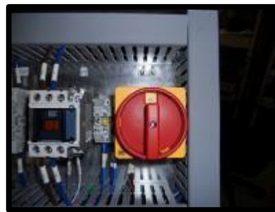
Figure 12, Main Power Disconnect
