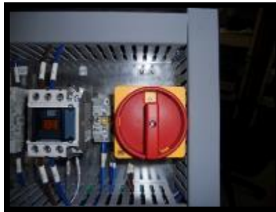
Main Power Disconnect
