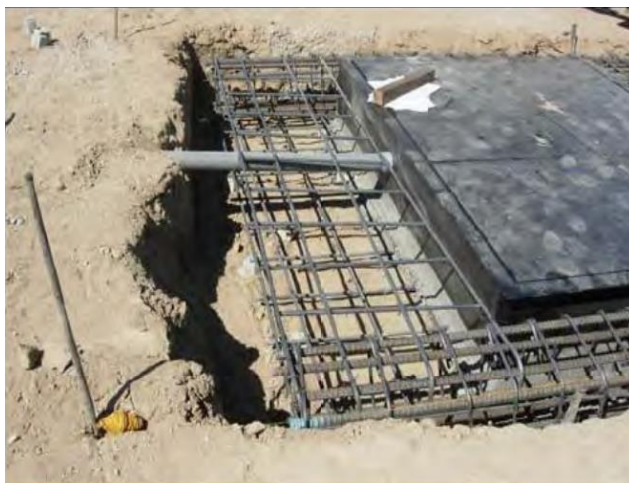
Picture 8 - Conduit Connection
